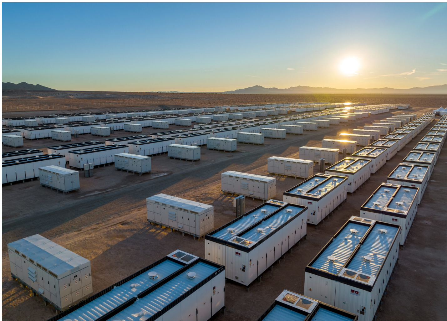
Recurrent's 1,400 MWh Crimson project in California | Image: Recurrent Energy
