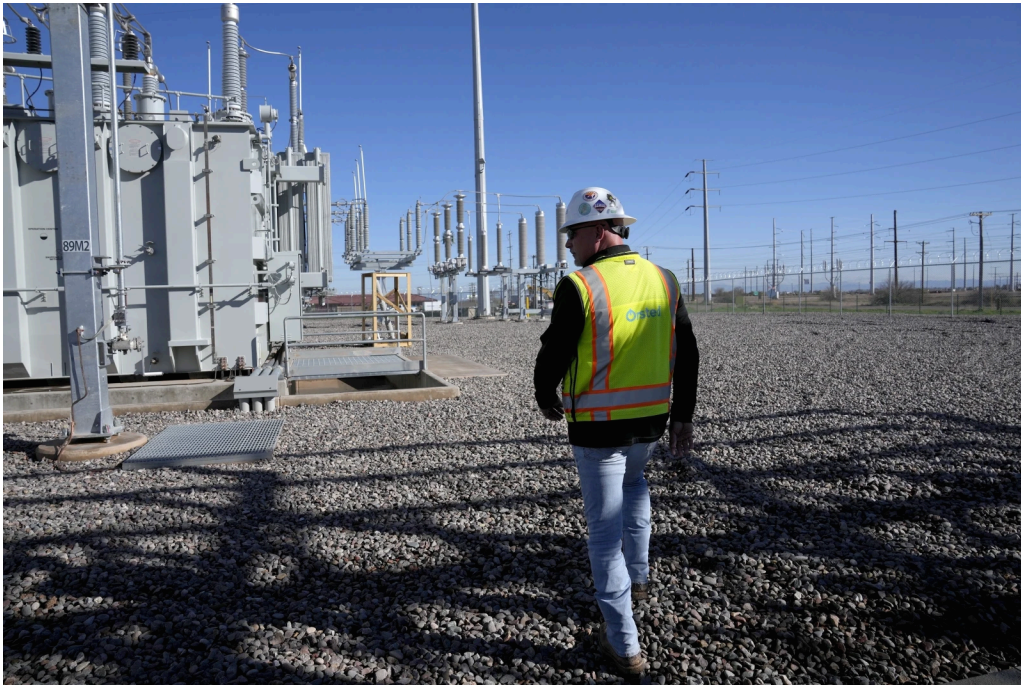
Mike Nutt, site manager, walks the campus at Orsted's Eleven Mile Solar Center lithium-ion battery storage energy facility Thursday, Feb. 29, 2024, in Coolidge, Ariz. (AP Photo/Ross D. Franklin) Read More
