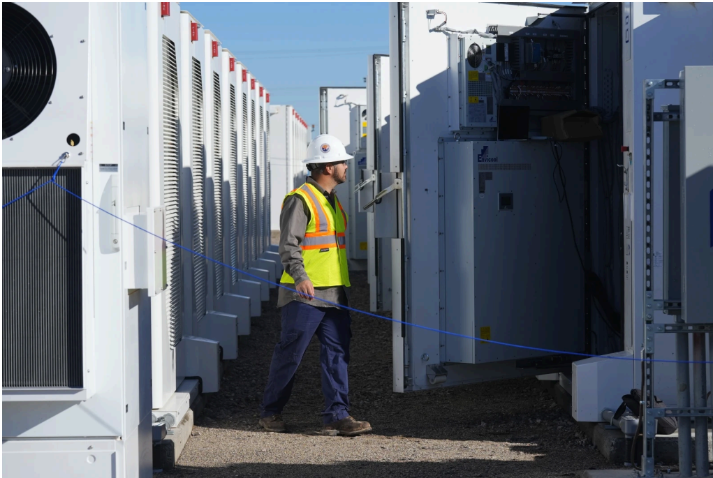
A worker does checks on battery storage pods at Orsted's Eleven Mile Solar Center lithium-ion battery storage energy facility Thursday, Feb. 29, 2024, in Coolidge, Ariz. (AP Photo/Ross D. Franklin) Read More
