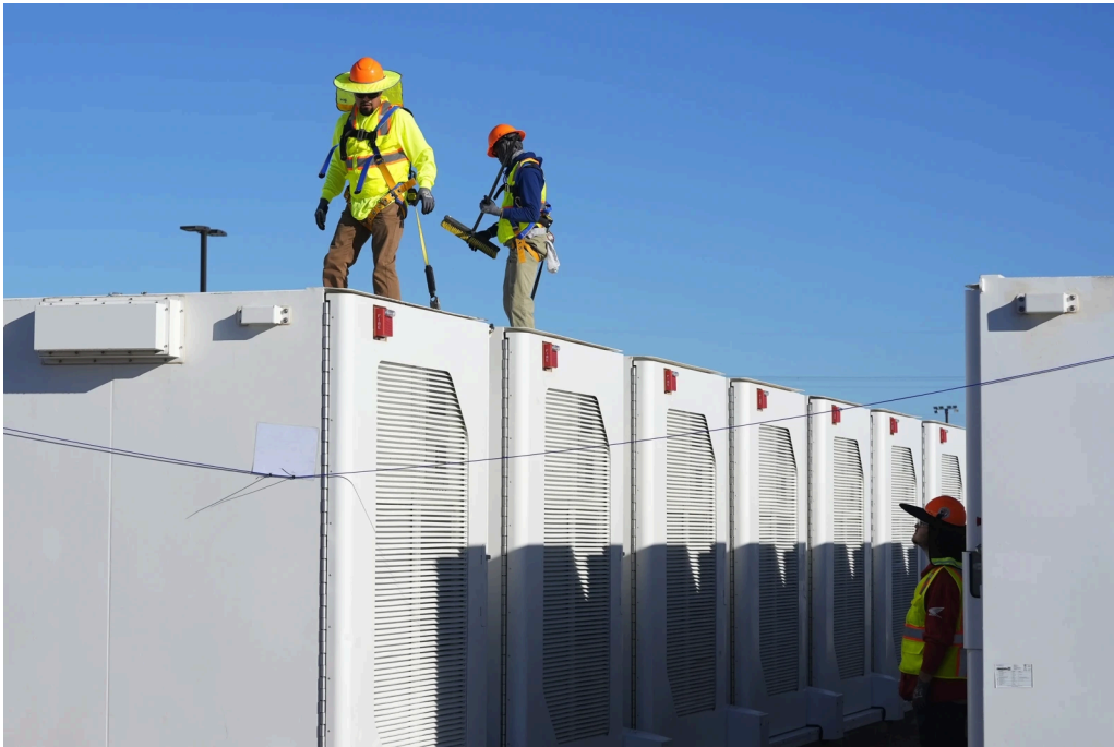
Workers do checks on battery storage pods at Orsted's Eleven Mile Solar Center lithium-ion battery storage energy facility Thursday, Feb. 29, 2024, in Coolidge, Ariz. (AP Photo/Ross D. Franklin) Read More
