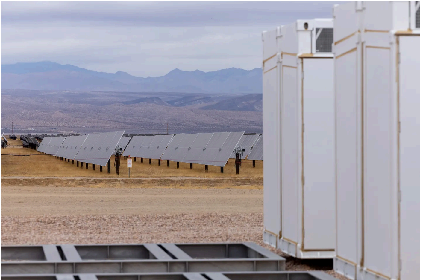
Battery solar energy storage units, right, at the Eland Solar and Storage Center in 2024. Brian van der Brug/Los Angeles Times via Getty Images
