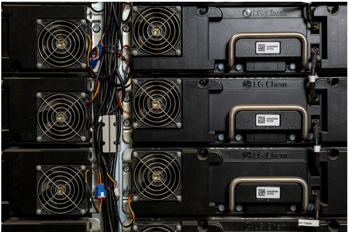
Lithium battery modules inside the battery building at the Vistra Corp. Moss Landing Energy Storage Facility in Moss Landing, California, in 2021. David Paul Morris/Bloomberg via Getty Images
